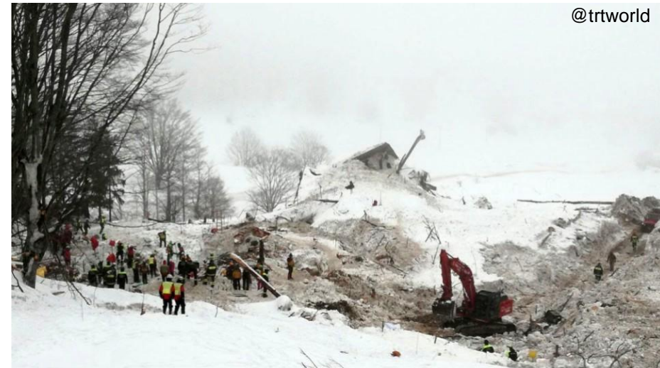
Destruction of an hotel by an avalanche in RigoPiano (2017), 29 casualties
