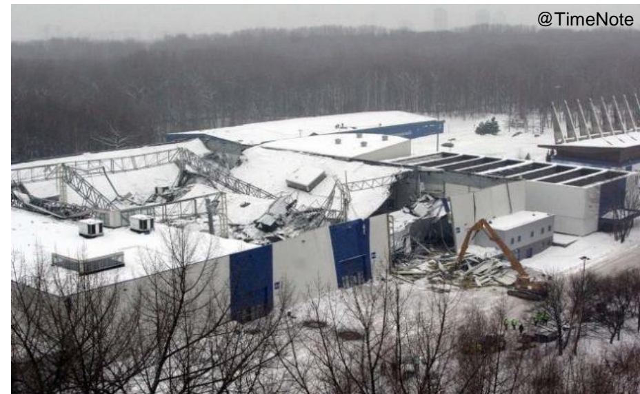
Roof collapse due to snowload, Katowice (2006), 65 casualties and 140 injured
