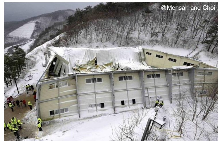
Roof collapse due to snowload, Gyeongju (South Korea) (2014), 10 casualties and more than 100 injured.
